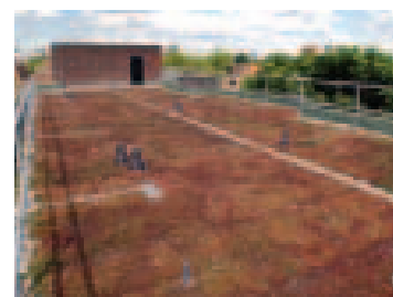
(Ethelred green roof, Ethelred Estate, Kennington, London. Source: Lambeth Council)
