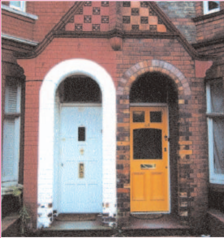
A fine original pair of doorways, the left one shows the unfortunate impact of painted brick work and an inappropriate door.
