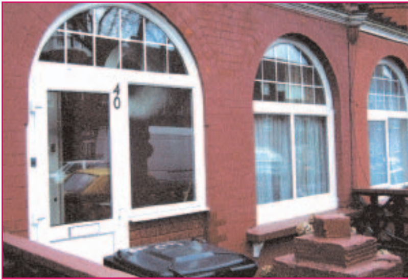
PVCu porch enclosure and inauthentic PVCu windows.
