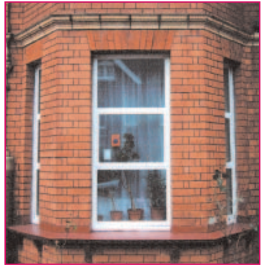
PVCu windows - with poor horizontal proportions.
