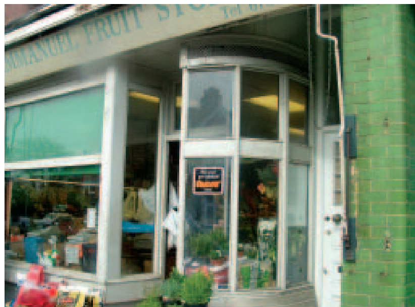
Fig 6: Altered shopfront retaining Edwardian joinery and glazed bricks
