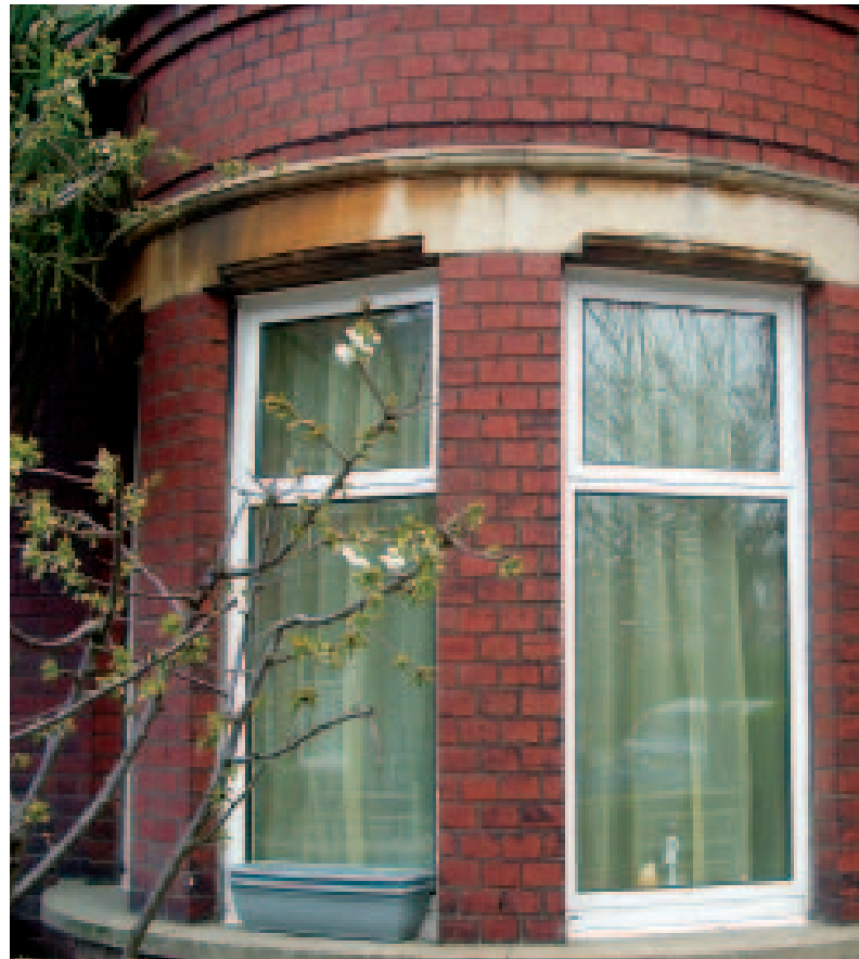
Fig 14: Aluminium replacement windows
