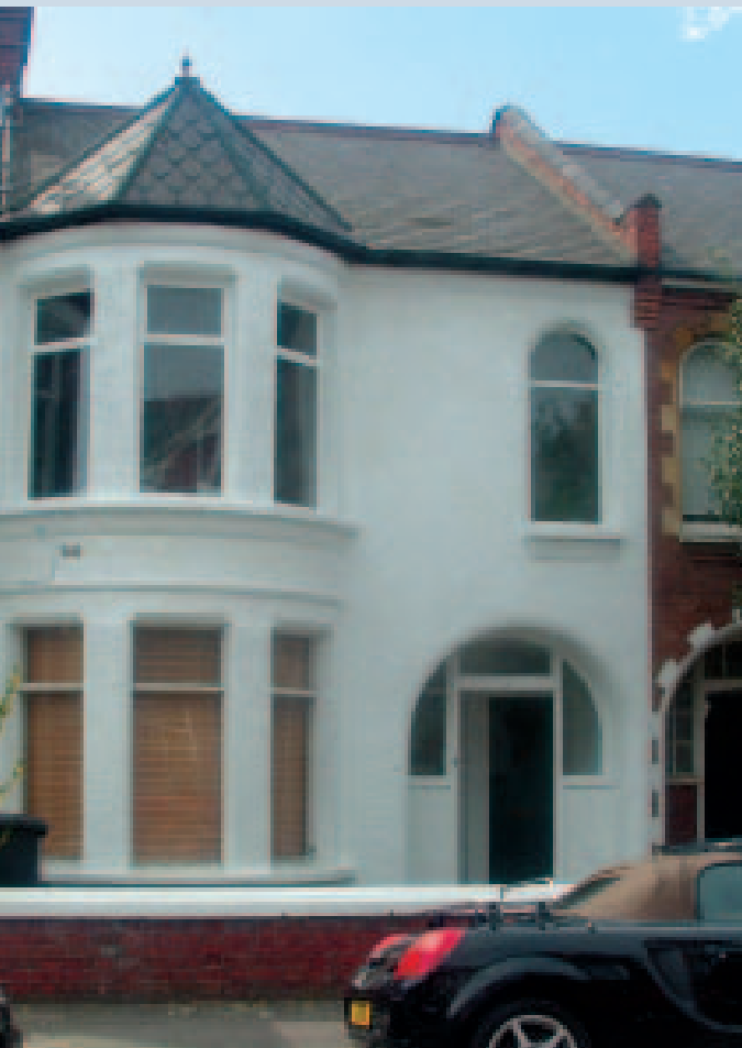
Fig 17: Brick detailing covered by render
