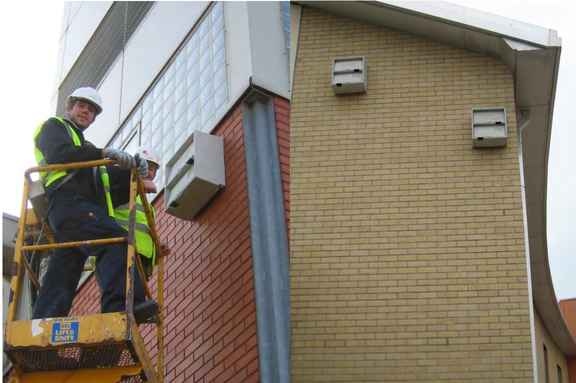
Plate 20. Erecting combined swift and bat nesting boxes on buildings at Lambeth Hospital, Landor Road, in partnership with South London & Maudsley NHS Trust
