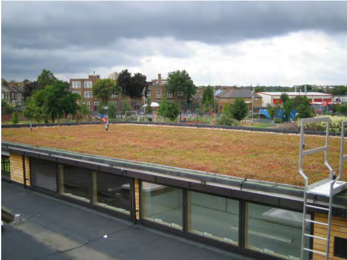
Plate 18. Part of the living roof on the Michael Tippett School, Herne Hill, which is still one of the largest green roofs on any school building in Greater London
