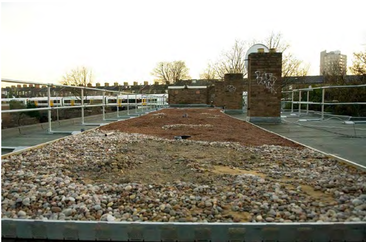
Plate 60. A new biodiverse living roof being constructed on the Fenwick Estate in Stockwell; the close proximity of a network of railway lines, as seen in the distance, was a key reason for its installation in order to extend and improve wildlife habitat
