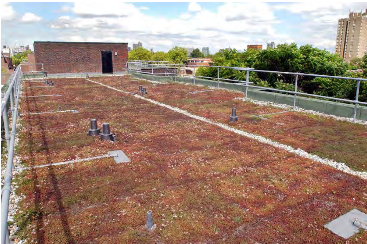
Plate 7. A mixed sedum species green roof on top of the Ethelred Estate in Vauxhall, which provides local biodiversity, flood mitigation and urban heat cooling benefits
