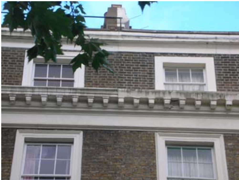
The crude stucco repairs (right) harm the appearance of the building.
