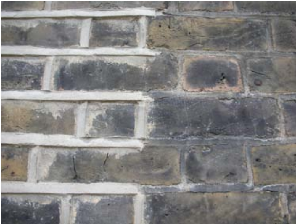
Poor modern 'struck' pointing in cement (left) should be avoided.
