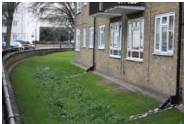
Figure 69 Example roof disconnections draining into raingardens at the foot of the estate (Source: SusDrain 29 )
