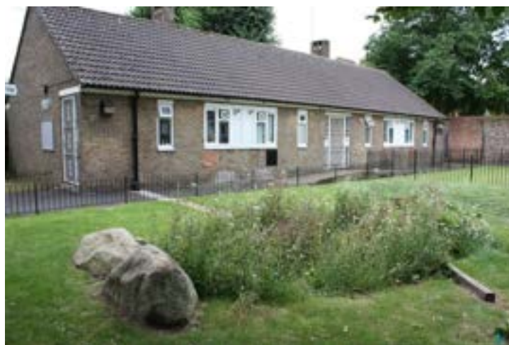
Figure 45 Example of roof disconnections draining into raingardens (Source: SusDrain 29 )
