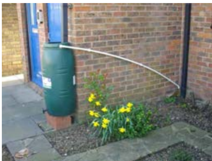
Figure 33 Example of a 100L water butt retrofitted to existing development
