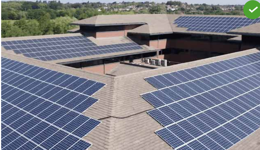
South-facing rooftop solar photovoltaic panels
