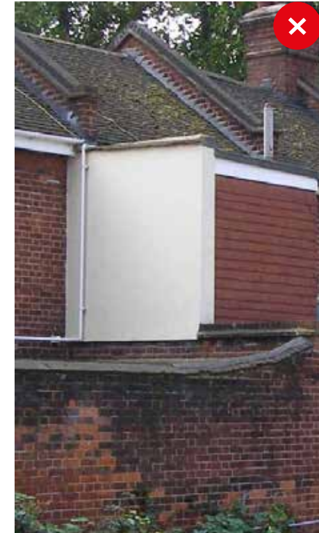
Unacceptable closet return
