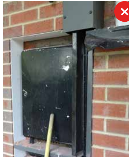
Risk of thermal cold bridging
