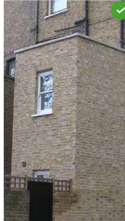
Acceptable closet return
