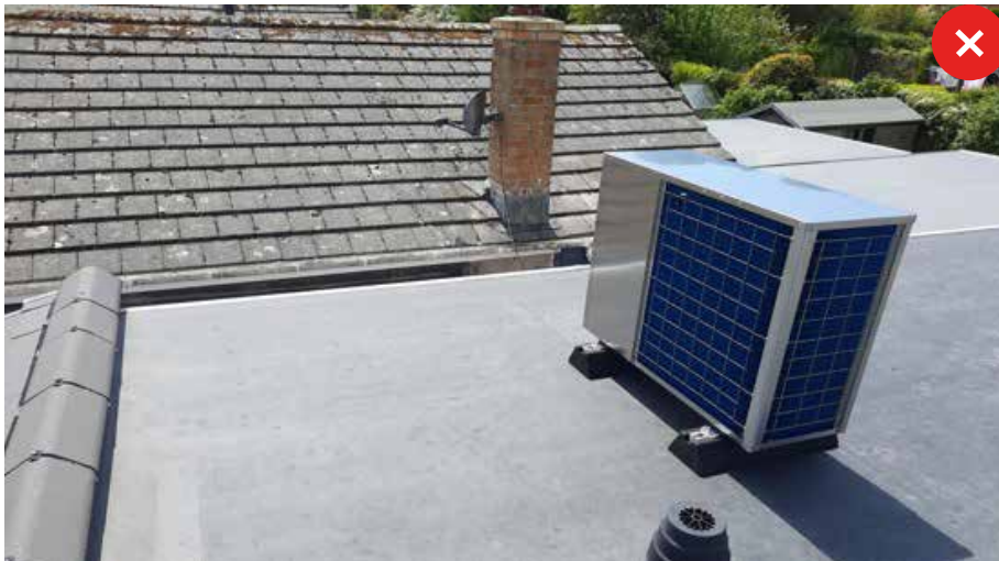
Visually intrusive locations should be avoided.
