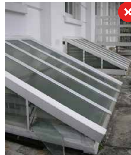
Glazing over light wells is not supported
