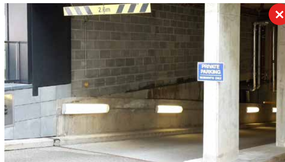
Poorly designed vehicular entrance.
