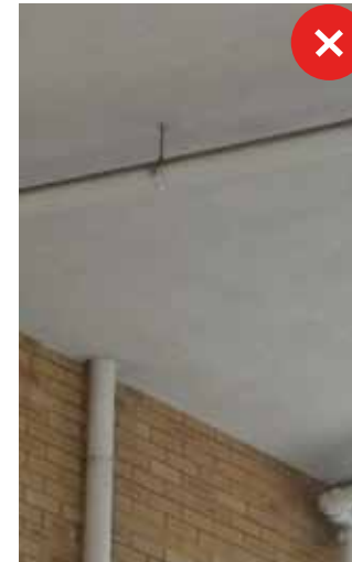
Soffit pipes unattractive
