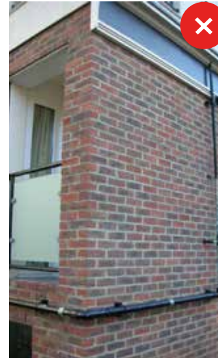
Ugly gas pipes
