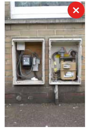
Damaged meter boxes
