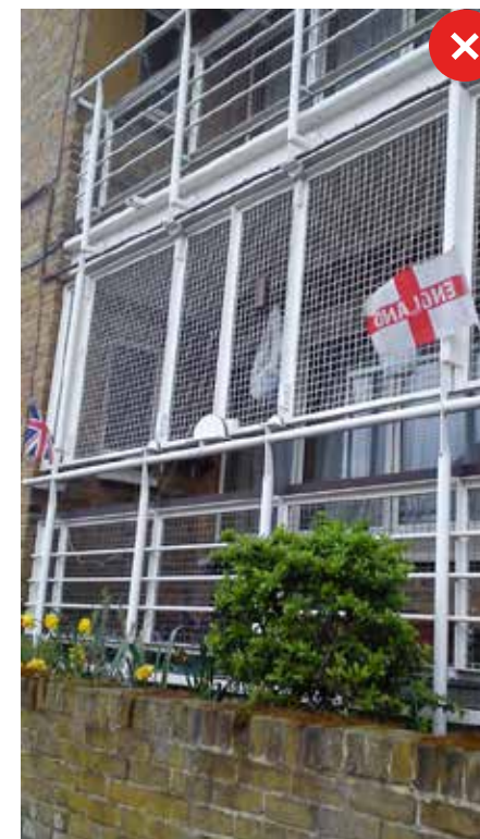
Caged balconies are unacceptable
