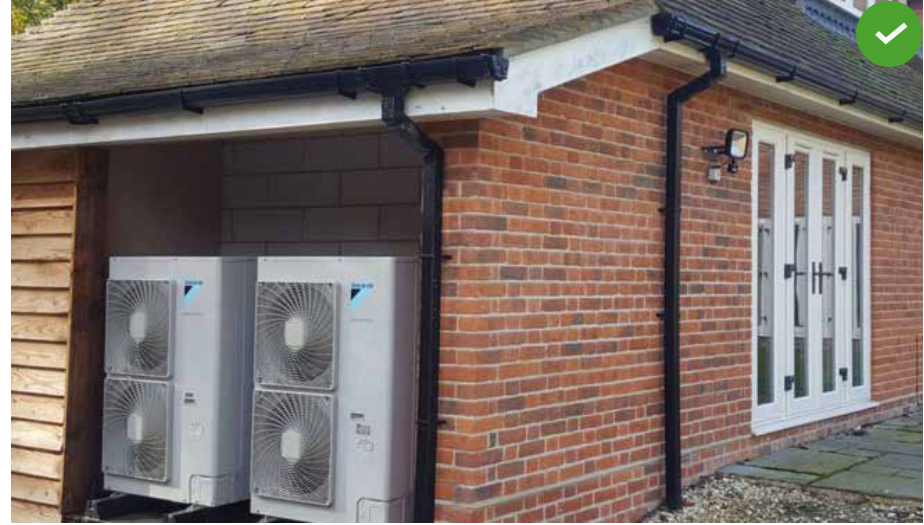
Heat pumps located within a considered enclosure
