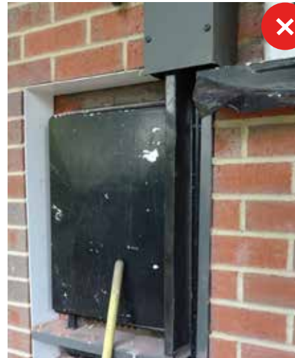
Risk of thermal cold bridging
