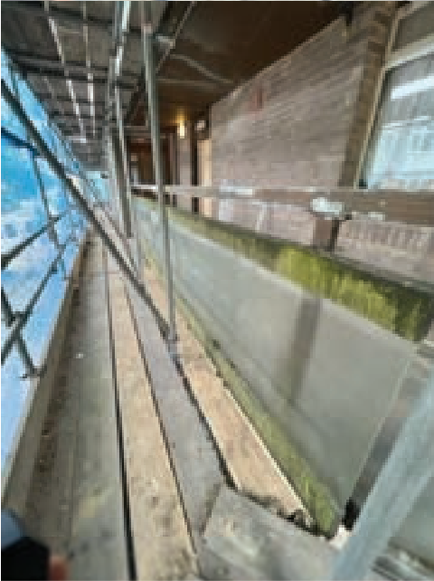
Left side: 6886 & 2907 & 5021 & 2950 & 5100 & 4900 Glass - 4th panel to be replaced - Cracked Repair Option – Replace Glass panel
