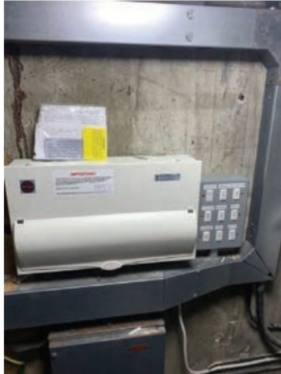
Baly house Distrubtion board
