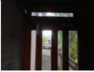
11.4 Fire door from the staircase to the balcony
