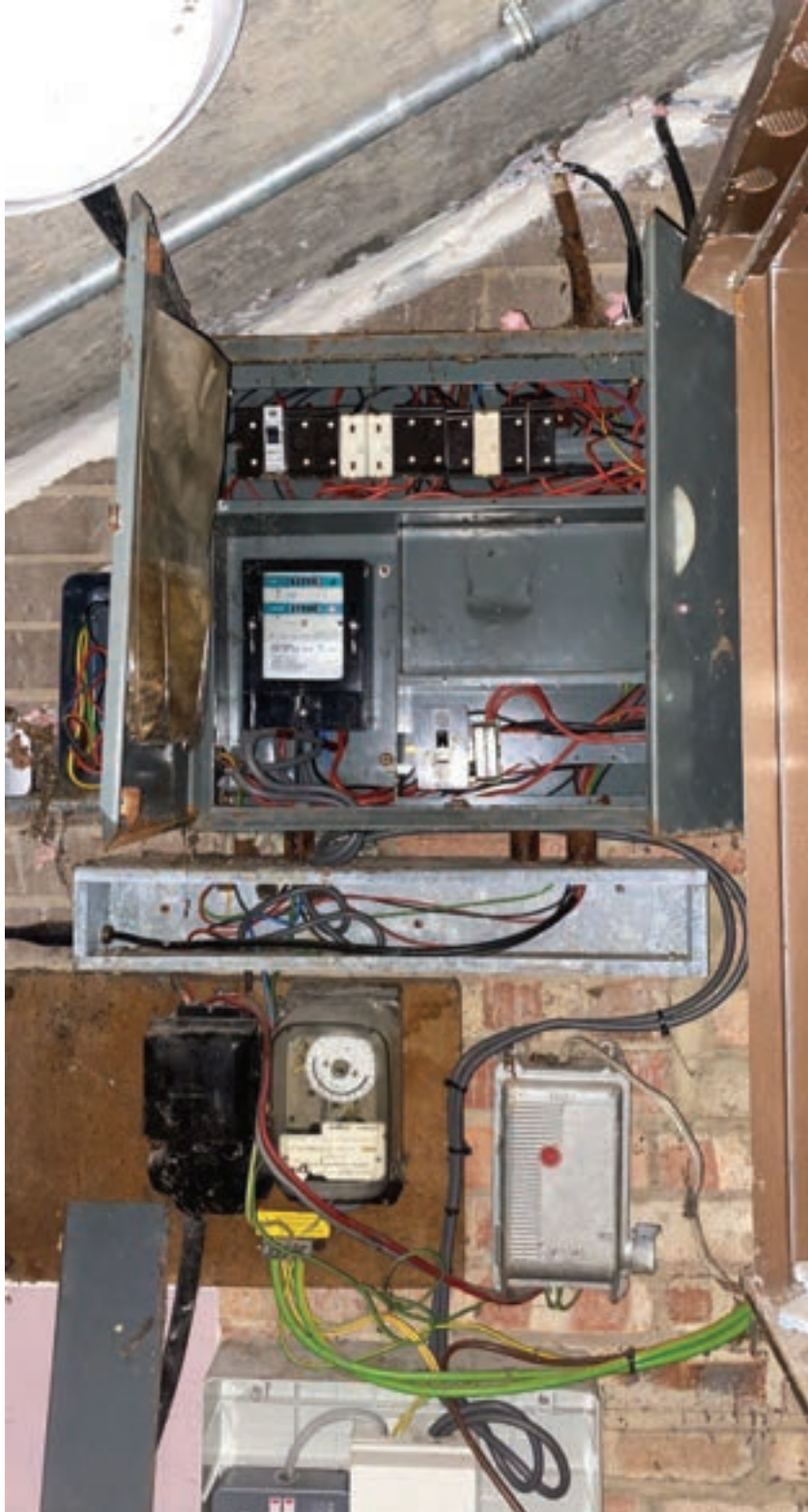
Chanler house Distribution board
