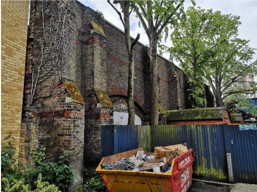
Figure 9 - The surviving section of boundary wall as viewed from the east. This eastern end is its tallest part of the wall. The western end is lower and plain.
