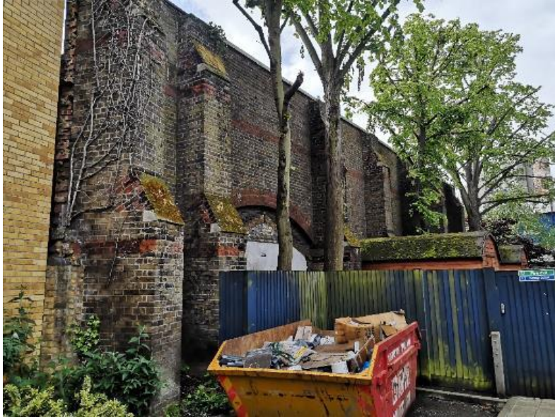
Figure 8 - The surviving section of boundary wall south of Wooden Spoon House as viewed from the east. This eastern end is its tallest part of the wall. The western end is lower and plain.
