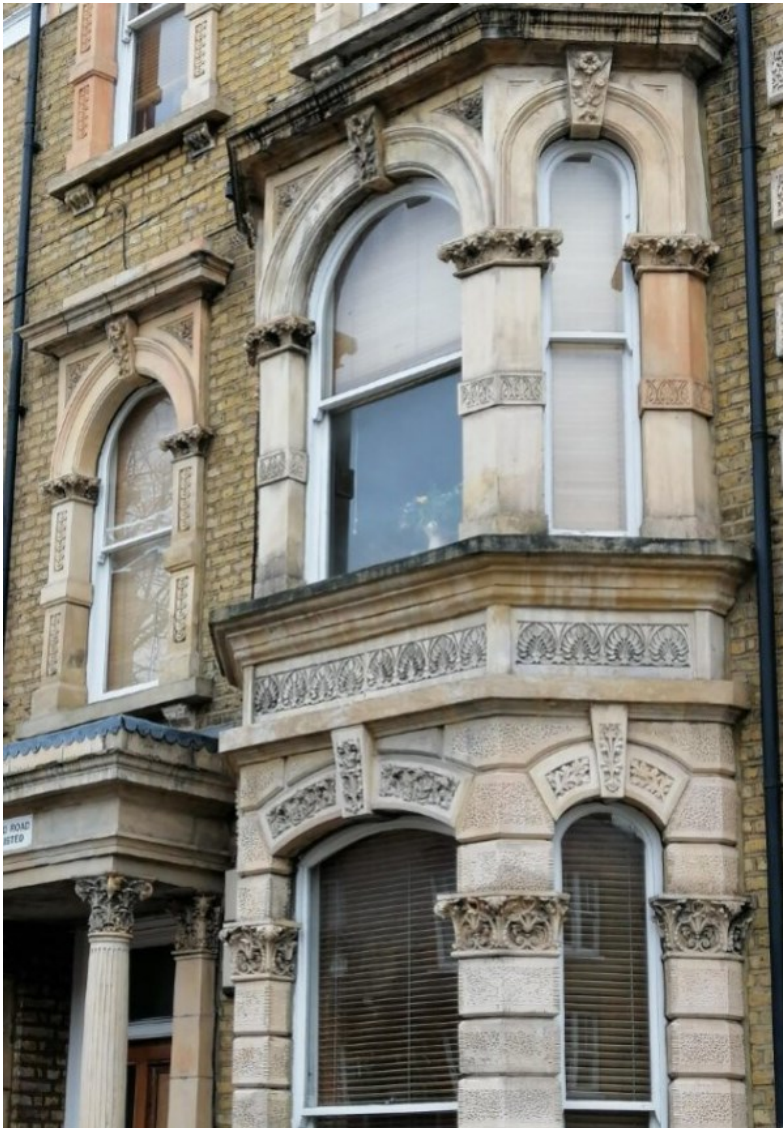
Figure 20 Authentic window and door detailing is a key aspect of the special interest of the area.
