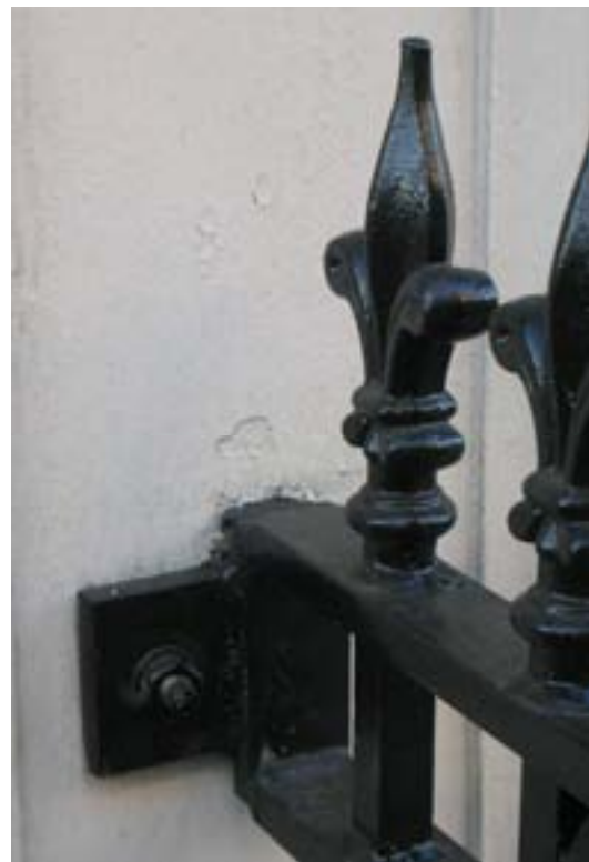
Right - Obtrusive brackets and visible bolts should be avoided
