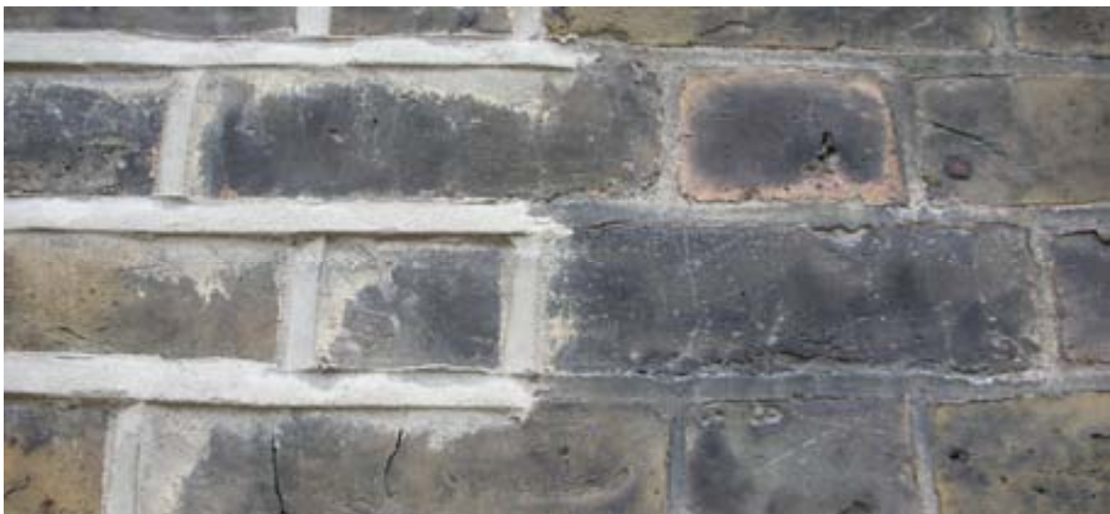
Weather-struck pointing in hard cement (left) harms the brickwork.
