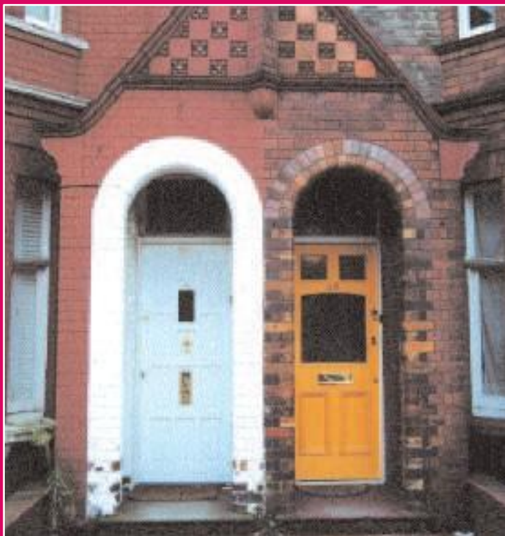
A fine original pair of doorways, the left one shows the unfortunate impact of painted brick work and an inappropriate door.
