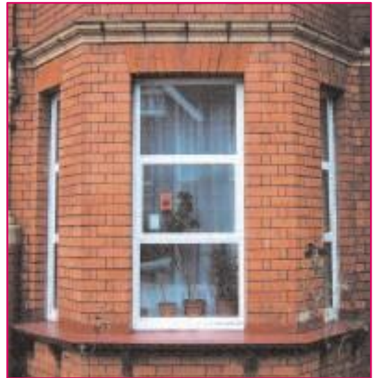
PVCu windows - with poor horizontal proportions.
