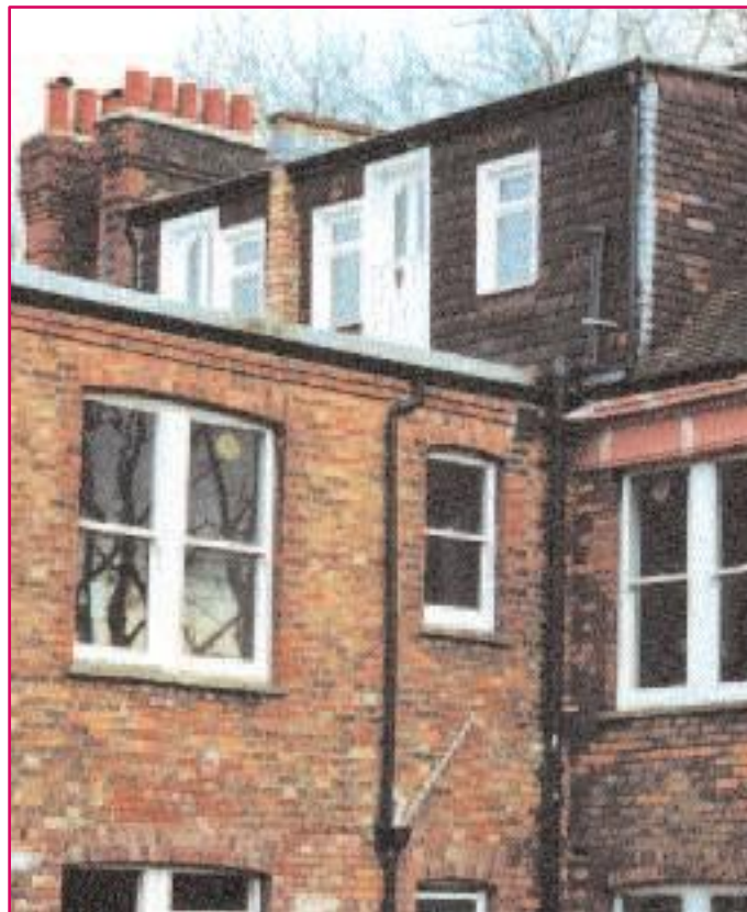
Inappropriate unauthorised bulky wide roof extension - subject to enforcement action.
