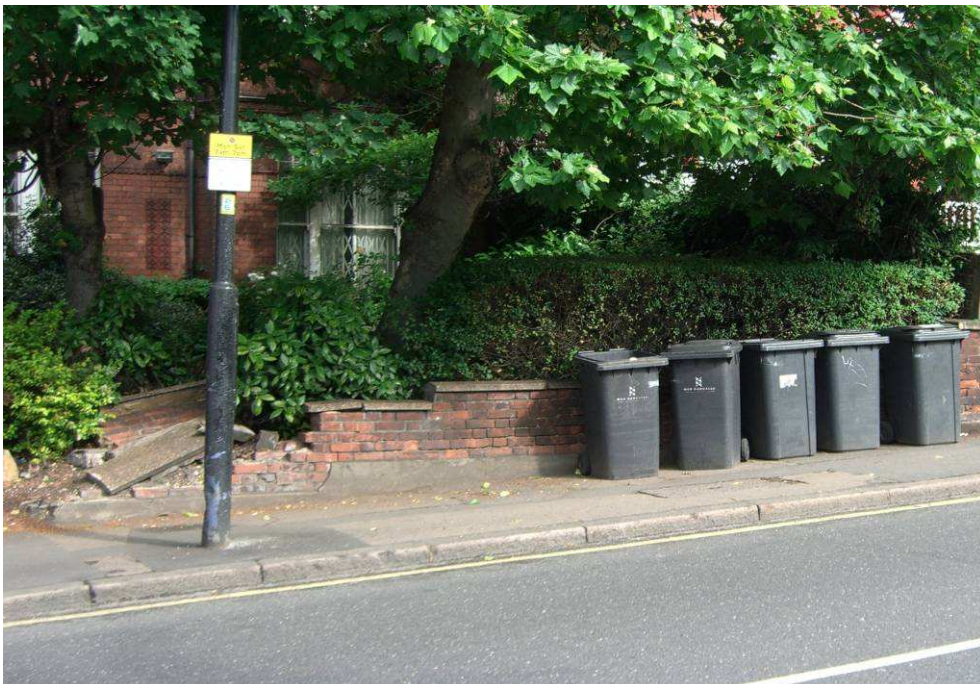
The dwarf wall at Herne Hill Mansions is in need of repair.
