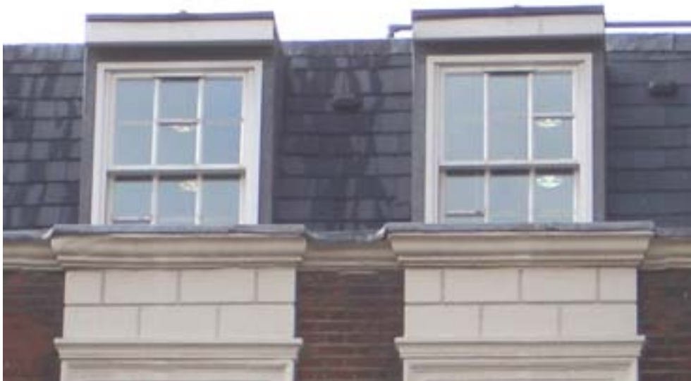
Stick-on glazing bars can drop off creating a poor appearance.
