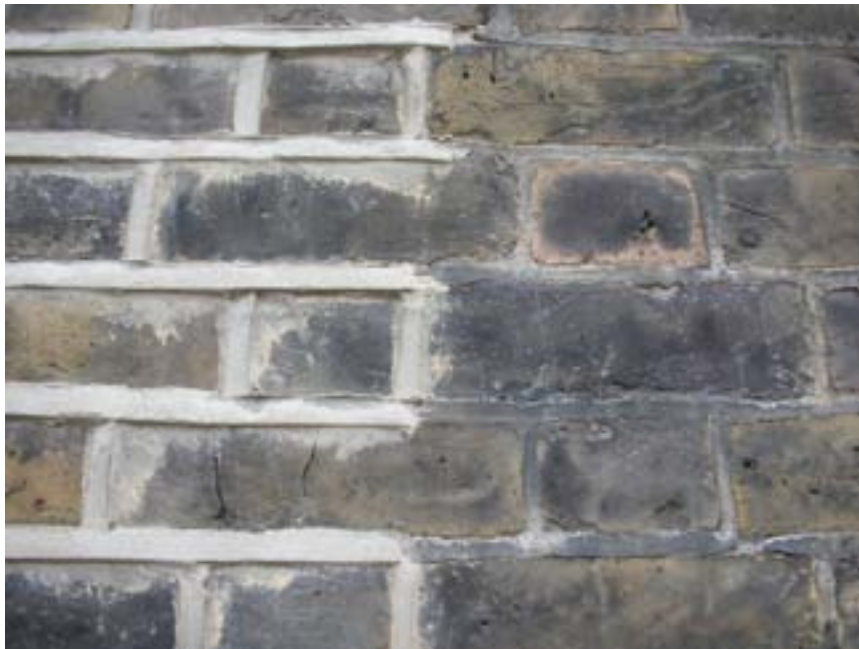
Modern tuck pointing in cement (left) is unacceptable.
