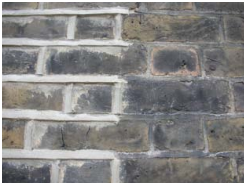
Modern cement pointing (left) harms the appearance of brickwork.
